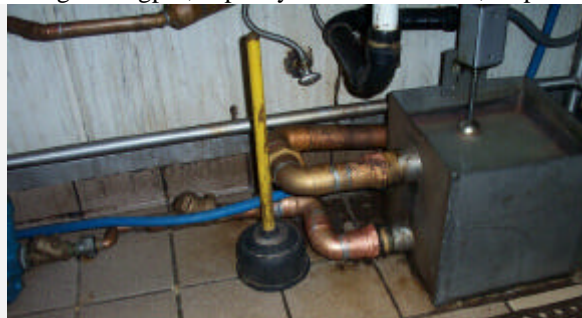
(f) Wastewater holding tank with automatic bypass
