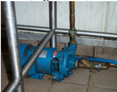
(e) Variable speed wastewater pump
